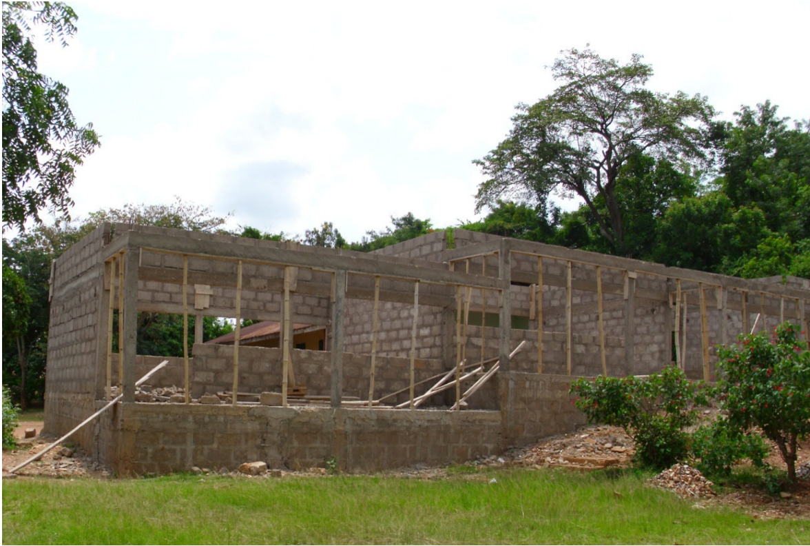
Construction of 6-unit classroom block with ancillary facilities at Peki-Blengo E.P. Primary School
