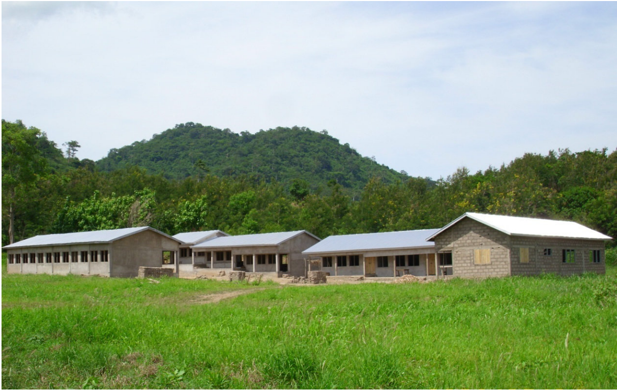
Construction of 6-unit & 3-unit classroom blocks with ancillary facilities at Kpeve Model School
