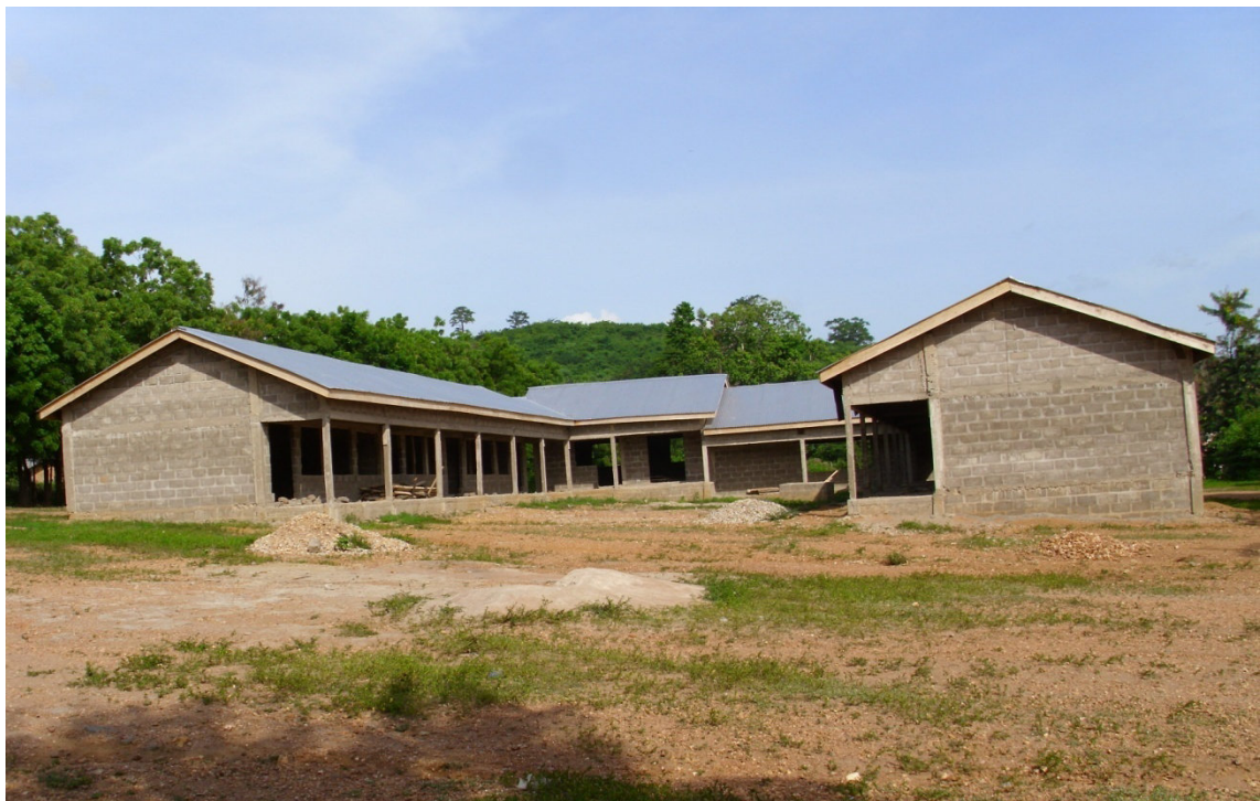
Construction of 6-unit classroom block with ancillary facilities at Tsatee E.P. Primary School
