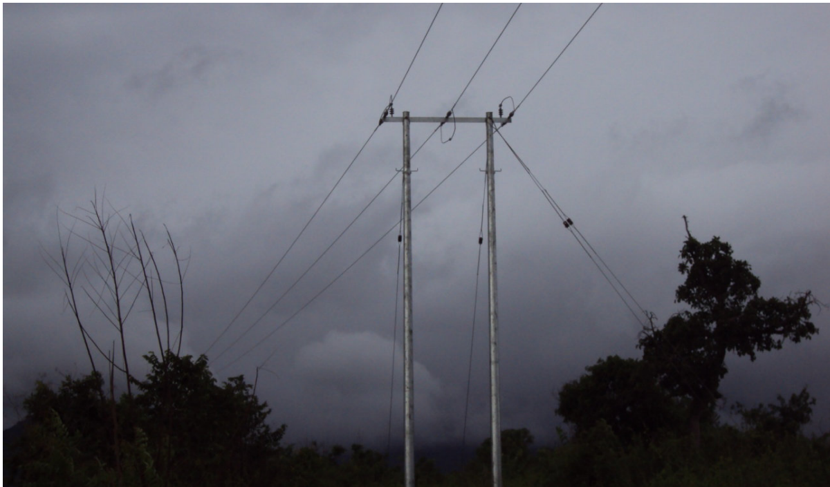
Extension of electricity to Fantekope, Abui-Tsita, New Kaira, Tsyokpokope, Kpeyiborme, Ayensu, Wawase, Wegbe-Camp, Kponkponikope, Gblorkope & Others under the Rural Electrification Project
