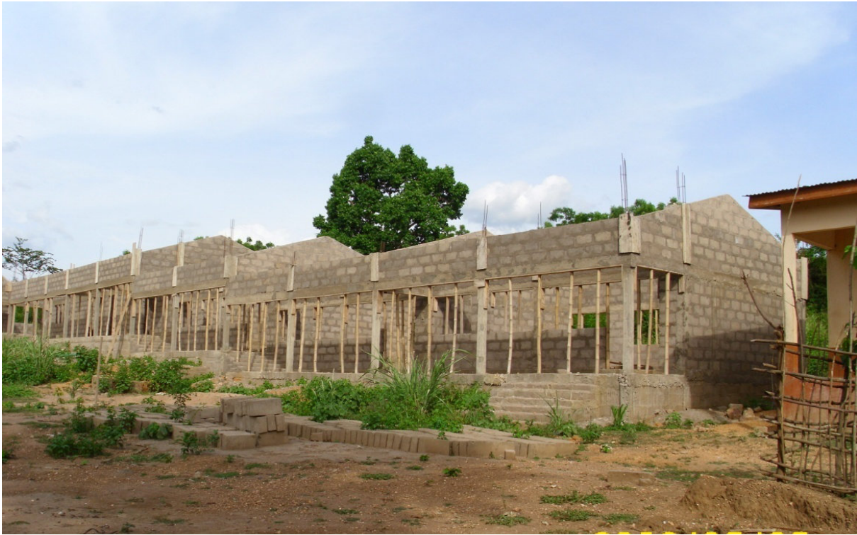
Construction of 6-unit classroom block with ancillary facilities at New Kaira LA Primary School
