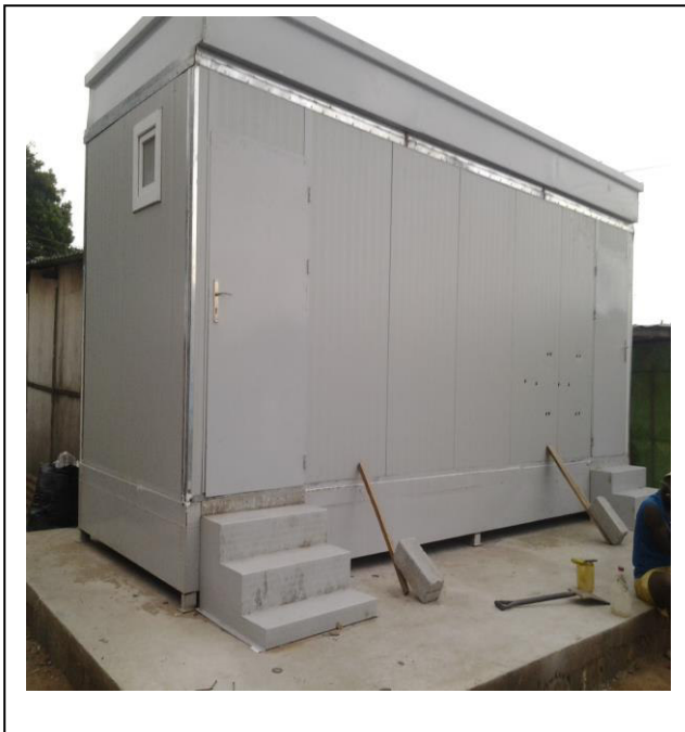
3. Mobile toilet being piloted at Tema Manhean
