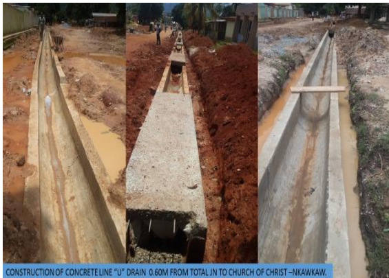
CONSTRUCTION OF CONCRETE LINE "U" DRAIN 0.60M FROM TOTAL JN TO CHURCH OF CHRIST--NKAWKAW. UDG TYPE 3. CONTRACT SUM: 190,000.00 STATUS: 100% COMPLETE
